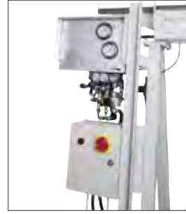
Detail of the control panel.
